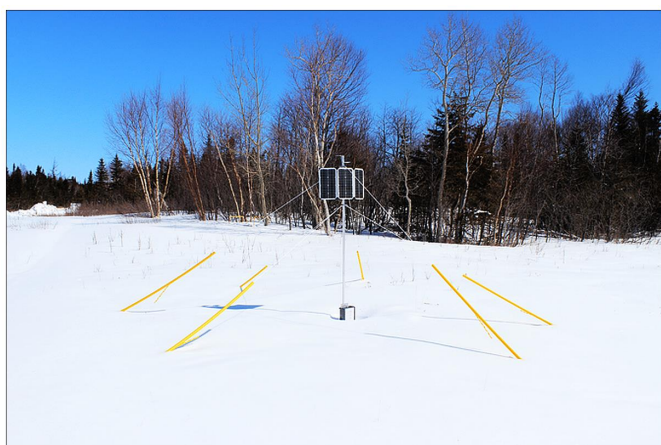
Autonomous station Installation in Newfoundland/Canada
